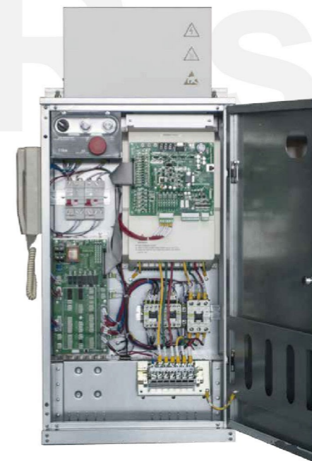
Machine room 机房
